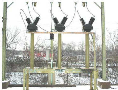
Fig. 21. 26 kV Potential Transformers
