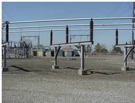
Fig. 12. 138 kV Open Air Bus on Post Insulators
