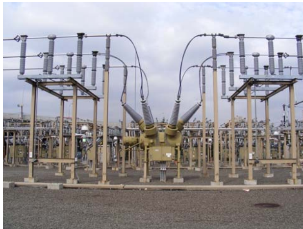
Fig. 5. 230 kV Outdoor 2000 A Circuit Breaker
