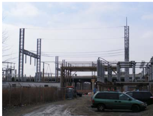
Fig. 14. 230 kV Strain Bus on Steel Towers
