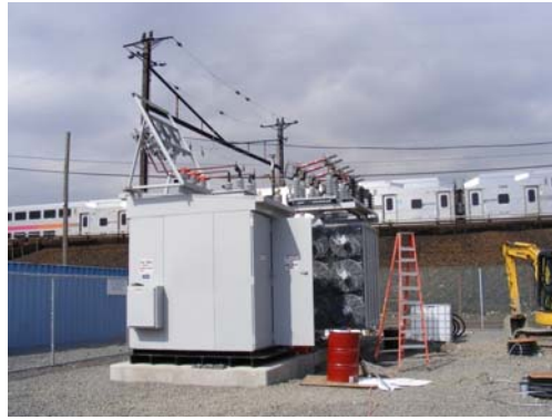
Fig. 25. 26/13 kV 9.0 MVA Unit Substation
