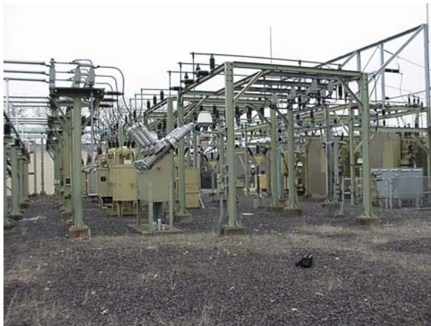
Fig. 6. 26 kV Outdoor 2000 A Circuit Breaker
