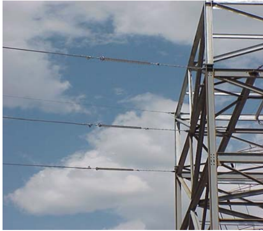
Fig. 15. 230 kV Strain Insulator Assembly
