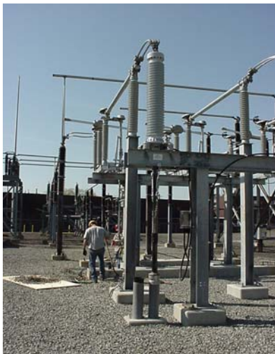
Fig. 17. 138 kV Solid Dielectric Cable Bus Terminal
