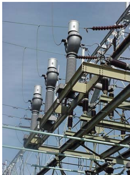
Fig. 18. Free Standing 138 kV 2000/5 A CTs
