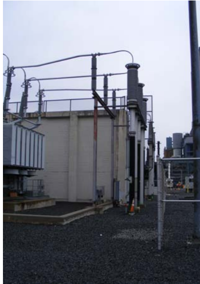
Fig. 16. 230 kV Gas Insulated Bus
